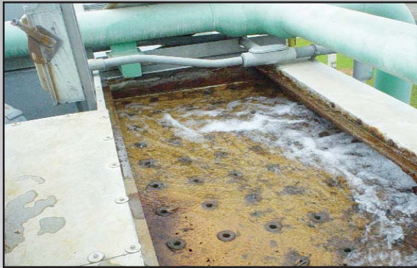
Marley NC Cooling Tower
